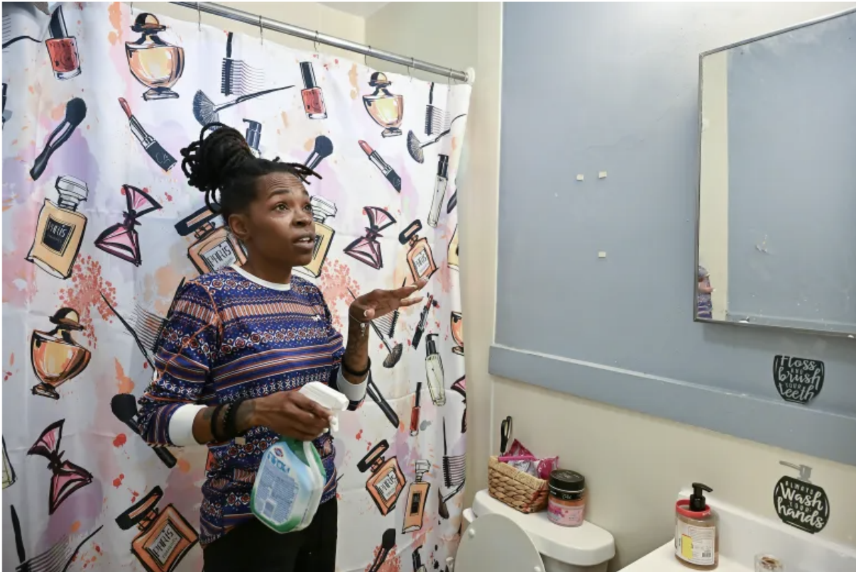
Eastport Terrace resident Heaven White talks about mold in her bathroom and the poor condition of the three Annapolis public housing units she has lived in over the years. (Paul W. Gillespie/Staff)
